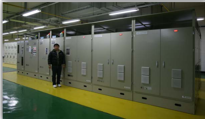
Operating ESS (City hall Substation)
