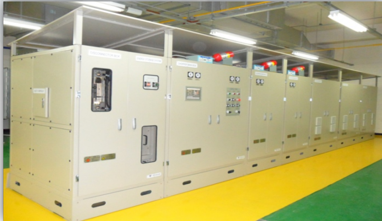
City hall Substation
